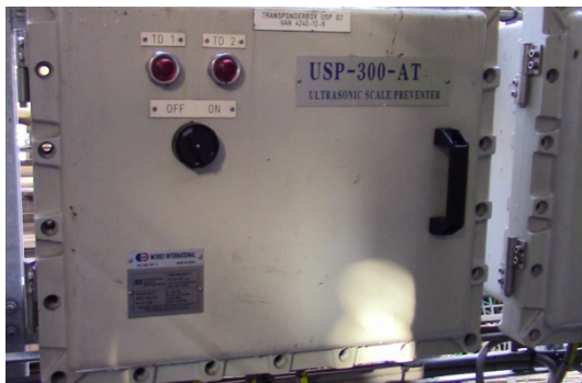
Fig. 4. One of the four, USP Ultrasonic Generators required for E-214A/B
