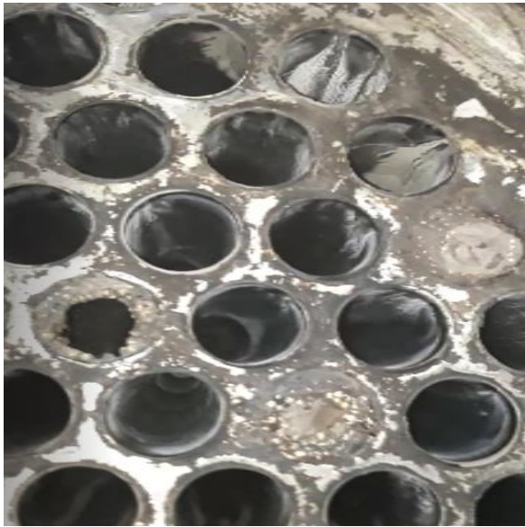
Figure 5: Inspection of the heat exchanger tubes of the first effect after 400 hours of operation
