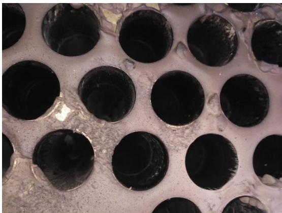
Figure 6: Inspection of the heat exchanger tubes of the third effect after 400 hours of operation
