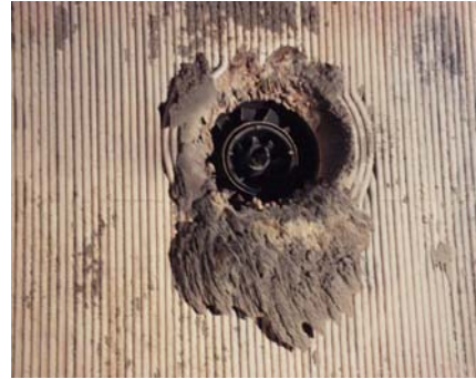
Fig. 14. Local slag deposit adjacent to the burner.
