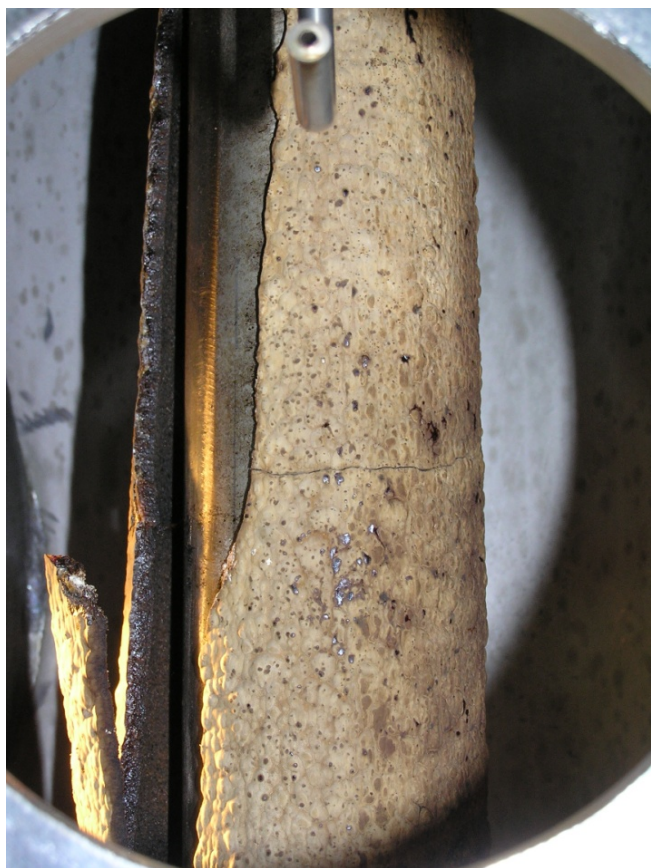
Fig. 4. Scales on the evaporator tube after an evaporator experiment (exp #3). Deposit thickness is around 5 mm.
