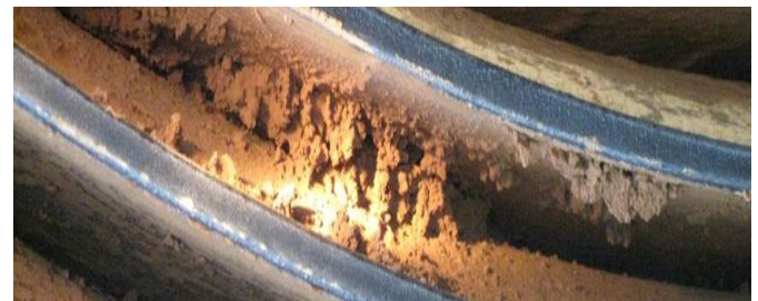
Fig. 5 - Close-up of Figure 2; heat exchanger with deposits.
