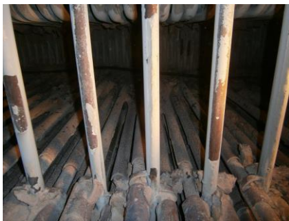
Fig. 4 Gap below RH II reheater – the area facing fly ash erosion hazard
