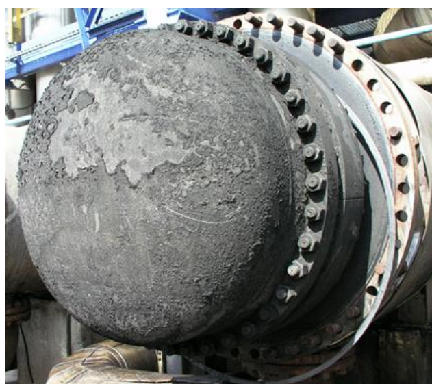
Fig. 6: Fouled heat exchanger (CDU preheat train)
