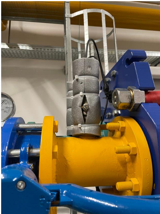
Figure 7: Insulation of valves to relieve the problem that the sensors measure the ambient air temperature rather than the temperature of the medias, on a customer installation.
